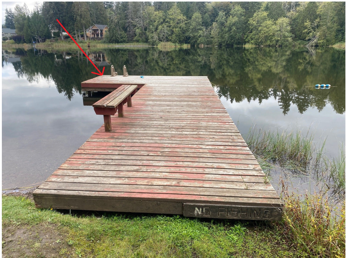
Dock #1 – Red arrow points to location of rotted (4x4") & cracked joist
