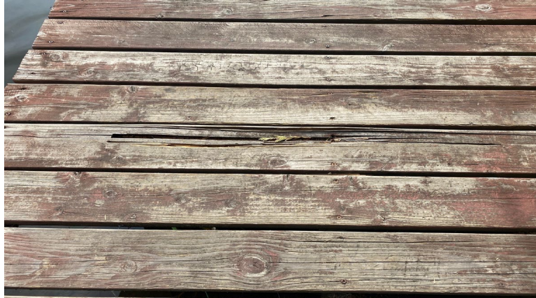
Dock #3 broken top deck plank
