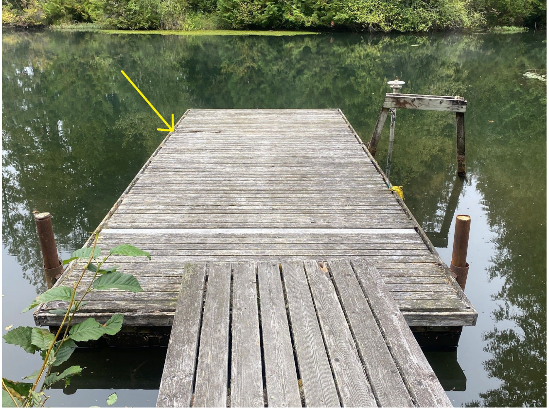
Dock #6 – Yellow line indicates broken plank that needs to be replaced
