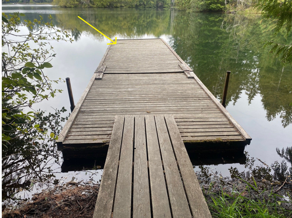
Dock #5 – The yellow line indicates the deck plank which is broken and needs replacing
