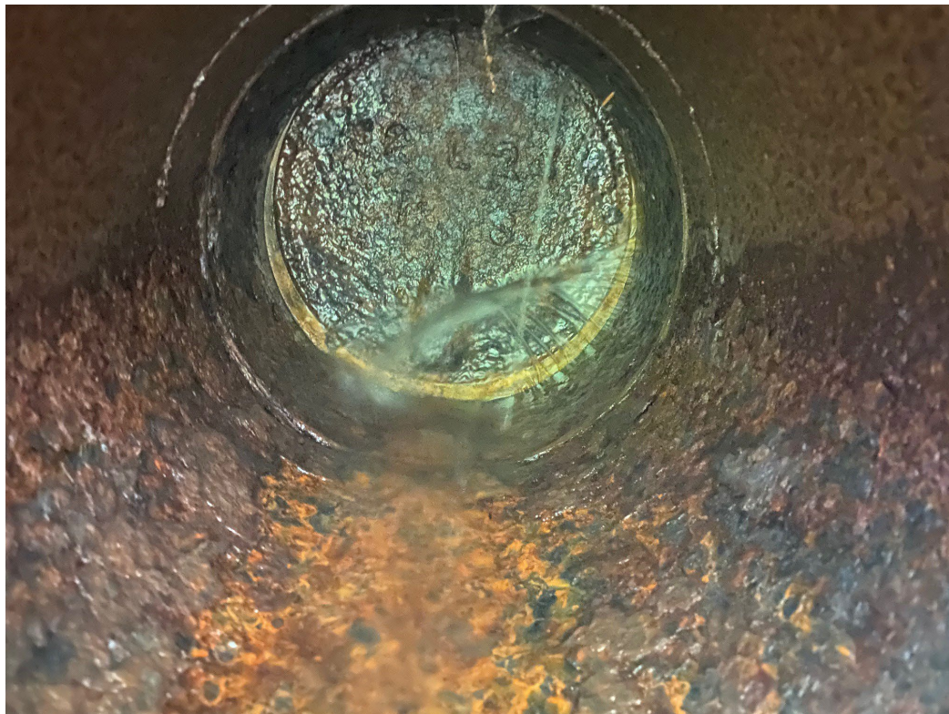
Lower valve water blow-by at 4 o'clock position after exercising valves
