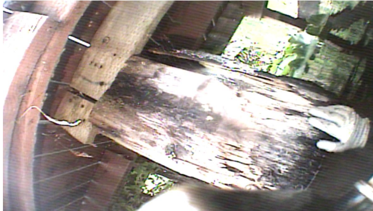
Dock #1 rotten stump supporting joist east side
