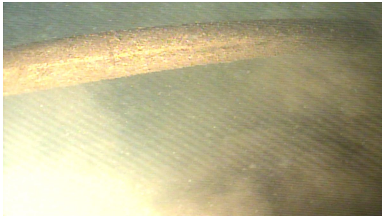
Dock #4 second galvanized steel piling condition
