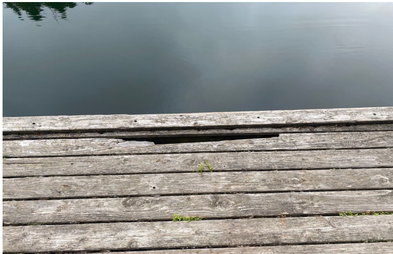
Dock #5 broken timber decking plank
