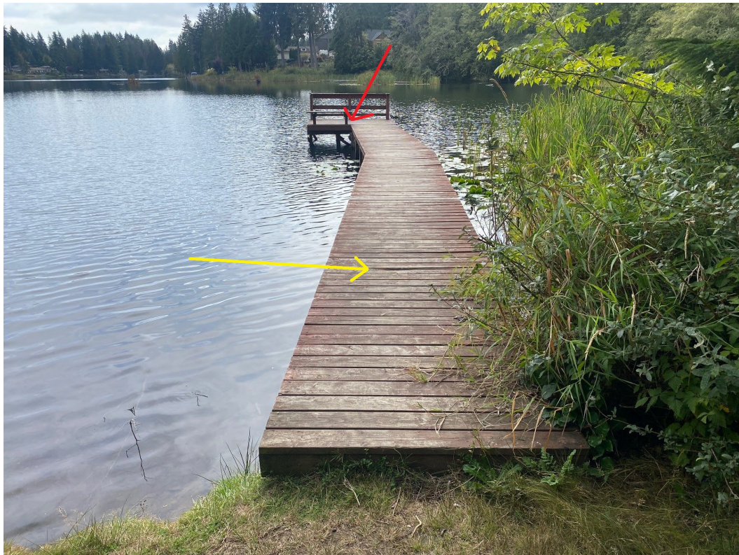
Dock #3 – Red arrow indicates area of rotted/loose cross brace, yellow arrow indicates area of broken top deck plank that needs replacing
