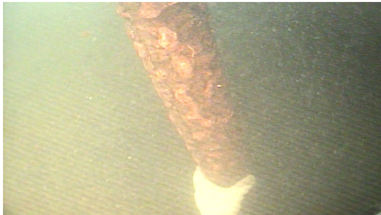
Dock #6 support piling with heavy rust & corrosion
