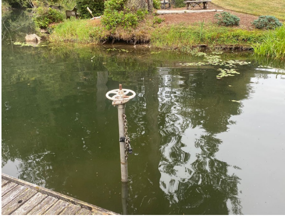
Upper sluice gate valve
