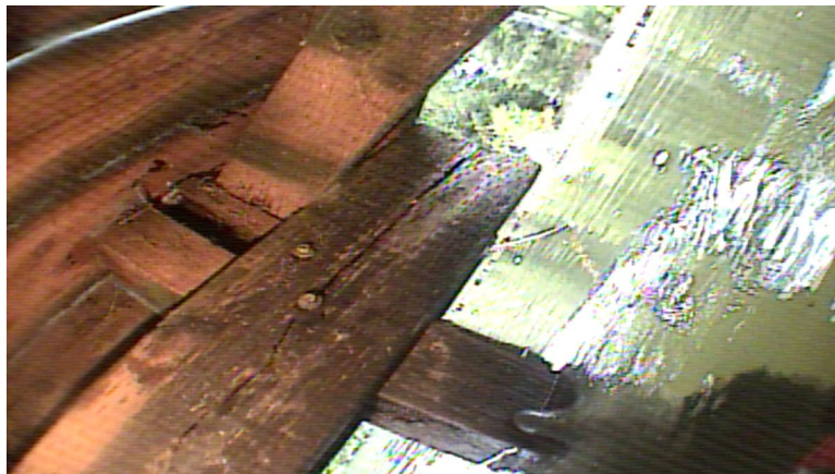
Dock #1 broken 2x6 joist southeast corner
