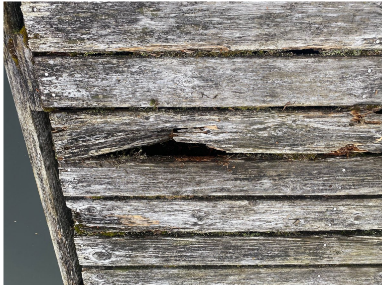
Dock #6 broken top deck plank
