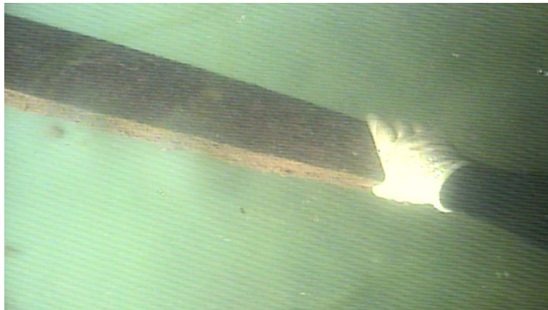
Dock #3 typical 4x4 support piling condition
