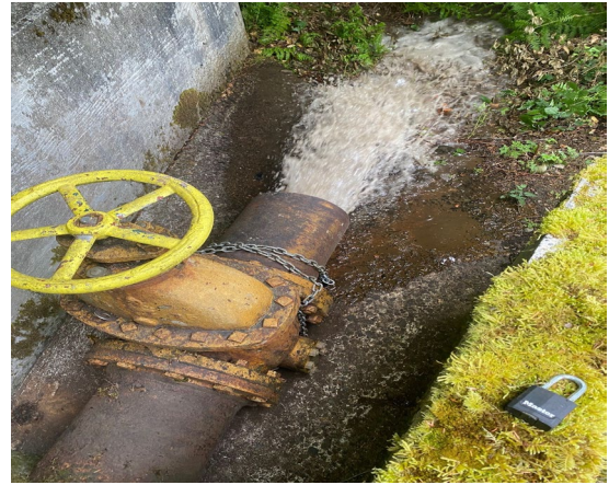
Lower sluice gate valve
