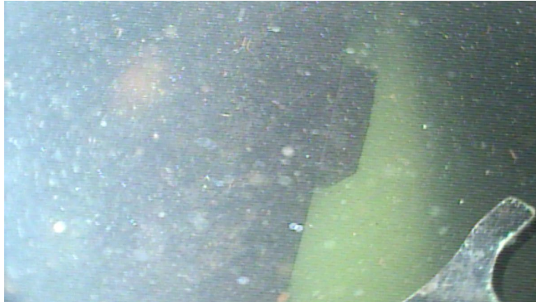
Dock #5 submerged timber condition
