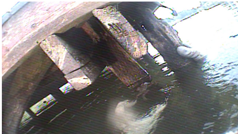
Dock #1 broken 2x6 joist southeast corner (view from South)
