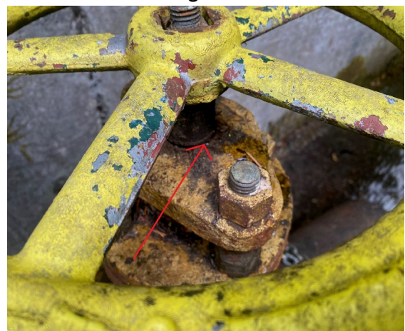
Leak from valve stem
