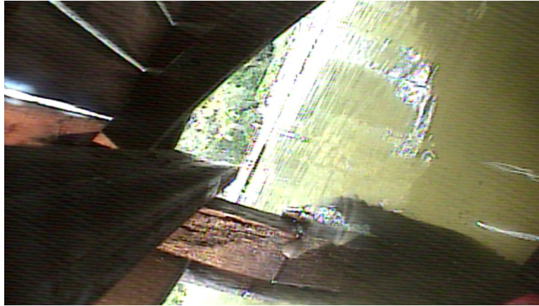
Dock #1 rotten 4x4 timber southeast corner
