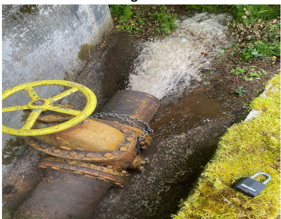
Lower valve open with upper valve cracked
